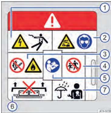
Fig. 141 Warning sign on high-voltage battery.
